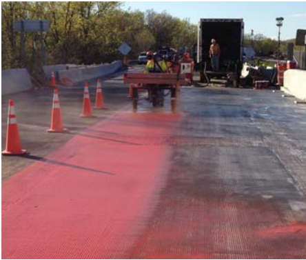
Spray Robot A worker monitors a spray robot applying 80 mils of BDM
