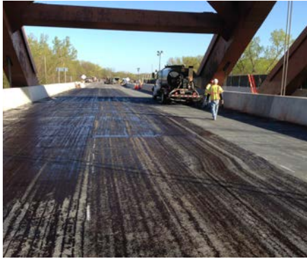
Tack Coat Application The asphalt wear course can be installed on the waterproofing system in as little as one hour
