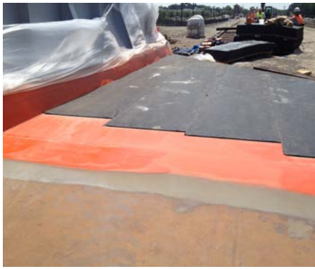
Protection Board Installation Workers began installing protection board immediately following the waterproofing installation.
