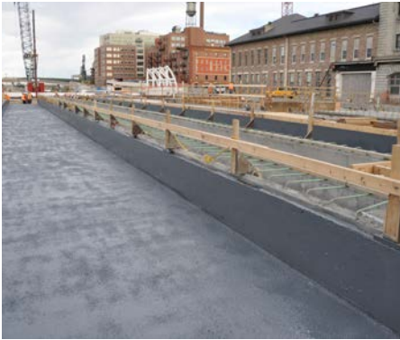
Completed System The bridge deck after Bridge Preservation™ Integrated Ballast Mat installation.
