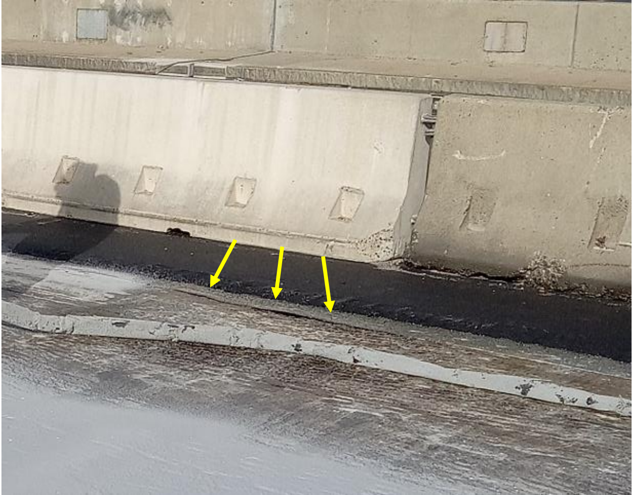
Improper Application Procedures & Techniques: Example of existing membrane that is not fully bonded to the substrate and can be defined as “unsound” in accordance with Section 2.2B above.
