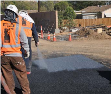
Partially Completed Installation Workers install the final seal coat of Integrated Ballast Mat.
