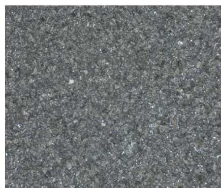
Finished Roadway Membrane A detail view of the finished roadway membrane system with aggregate.
