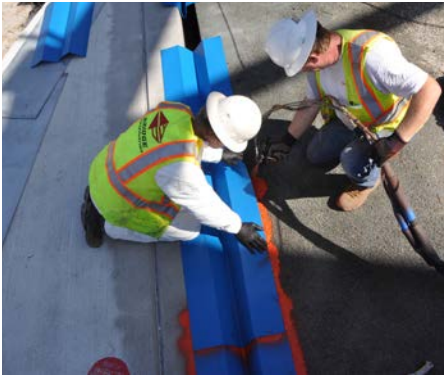
Articulus™ Expansion Joint Installation Workers install a section of the spray-applied expansion joint system.
