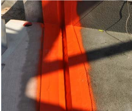
Completed Joint Installation The completed expansion joint installation at the north abutment prior to placement of the protection plate.
